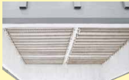
Heating elements in furnace hood
