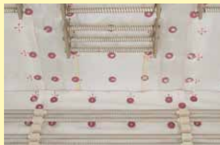
Fabric cover on the fiber roof (and sides) to reduce fiber dust
