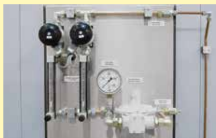
Gas supply system for non-flammable protective or reaction gases
